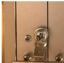
Picture 3-5-1-1 Earth connection point of the device at the Power supply module
