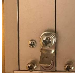
Picture 3-5-1-1 Earth connection point of the device at the Power supply module
